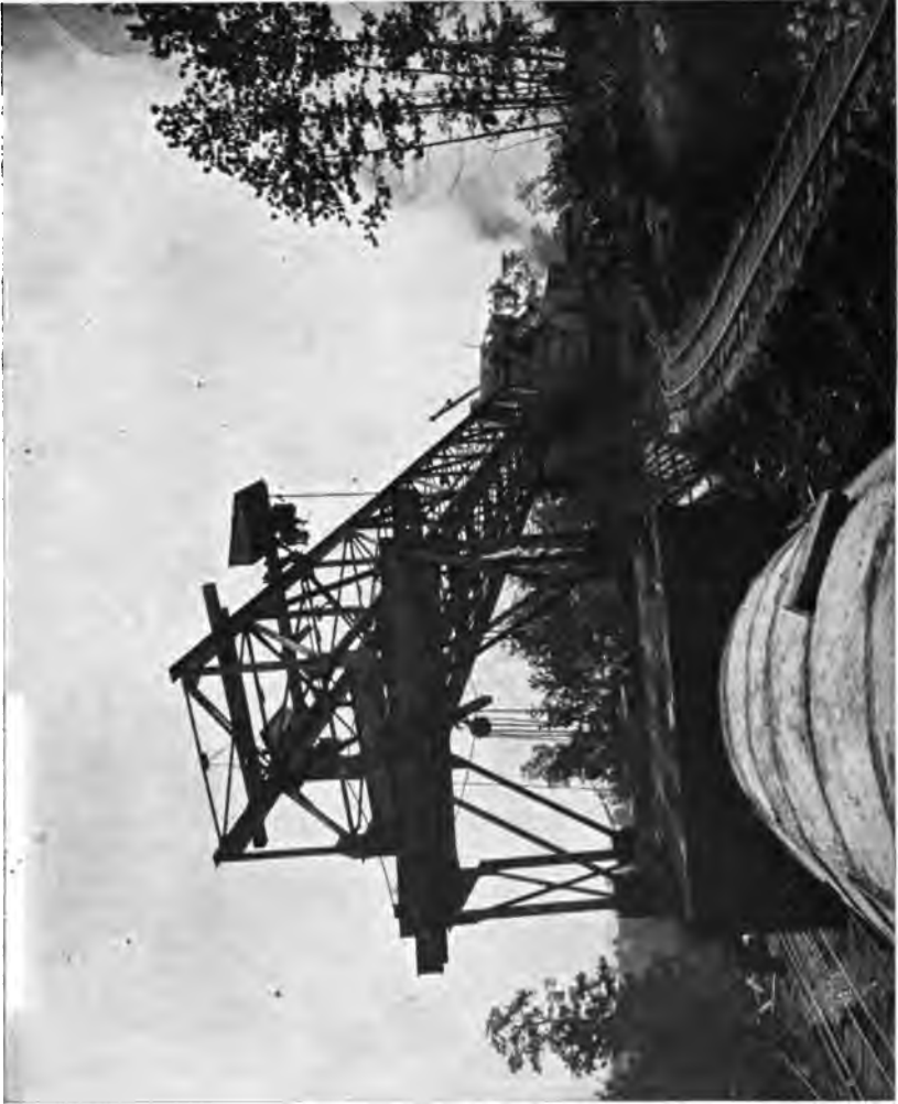
PLATE 67. —Contract 11. Traveling Crushing and Concrete Plant, Showing Saddles at Rear of Bridge and Bridge with Overhead Traveler for Moving Outside Forms.
